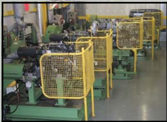
Header Tank Heat Exchanger Units on a production engine test facility.
